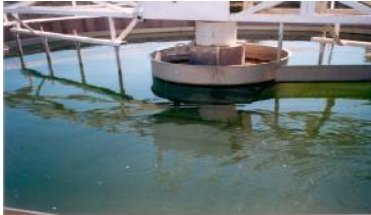
Figure 4: Wastewater treatment facility in one food processing company that is listed in the Green Book.
